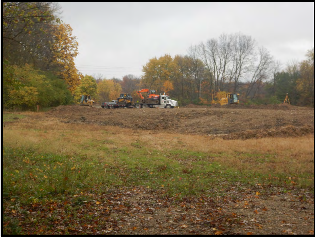
Figure 12. Disturbed conditions south of US 42.
