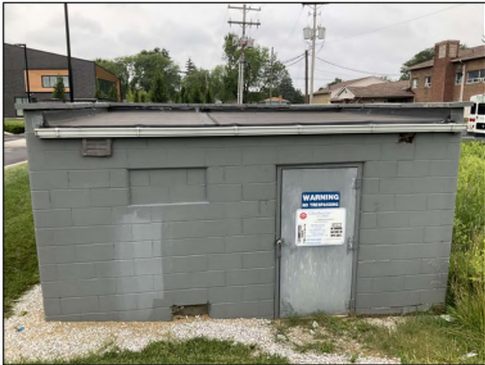
Photo 28: View of Karl & Cottonwood Station, facing north.
