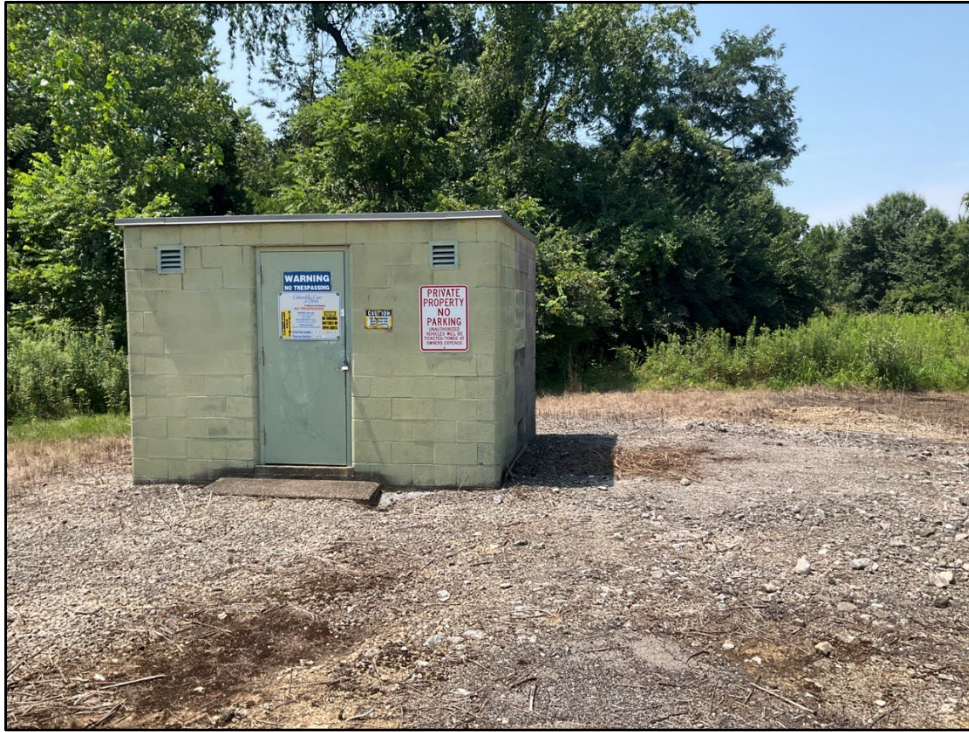
Photo 7: View of representative existing station on Sunbury Road, facing west.
